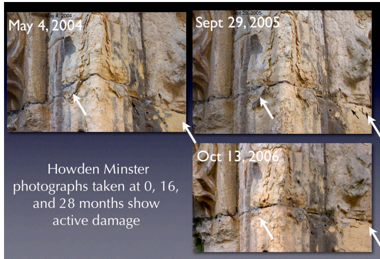
Figure 2. Results from repeat photography showing the creation of new flakes and the loss of old flakes over a period of 28 months documents active damage to Magnesian Limestone.
